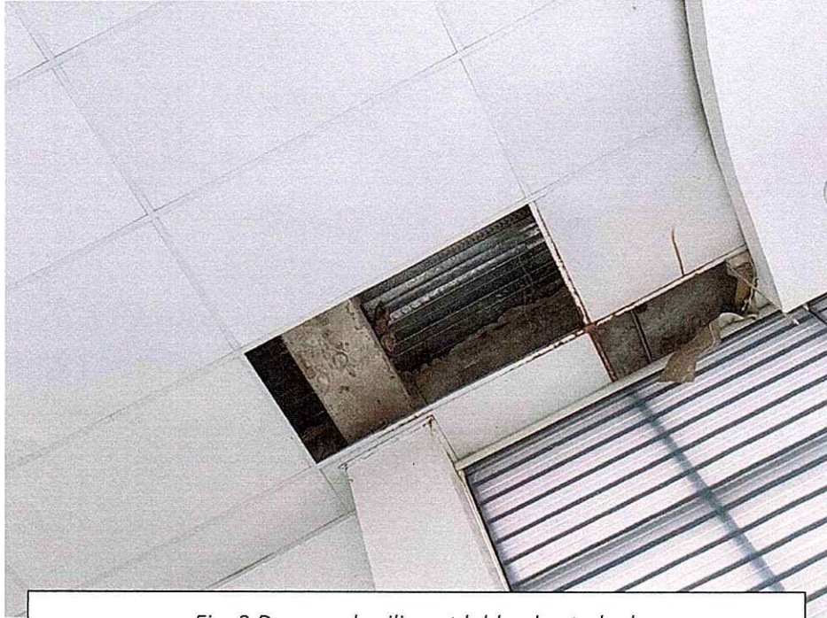
Fig. 3 Damaged ceiling at lobby due to leak
