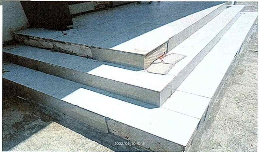
Fig. 1 Indication of a soil settlement as seen from the side entrance of the building
